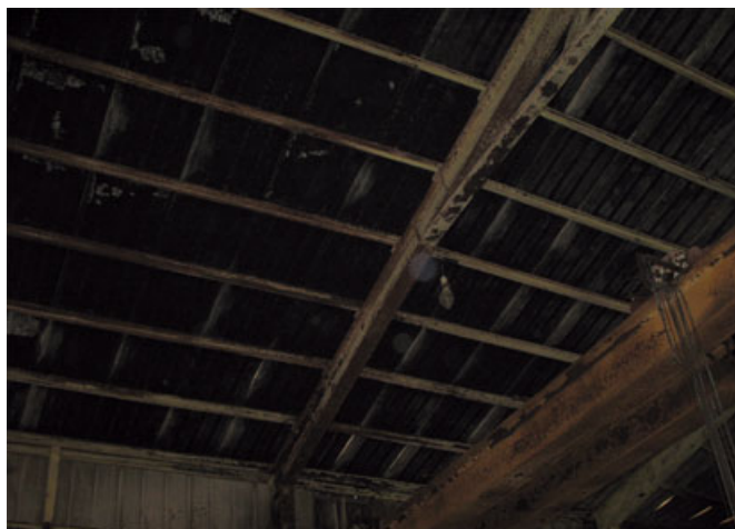
FIG. 6—Smoke damage of ceiling.
